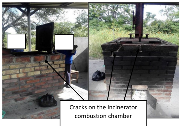
Fig. 28 Cracked incinerator used to dispose solid waste at ST Theresa hospital Source: Field data (2023)
